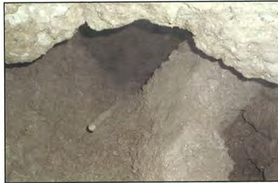
Excavation left of fallen rock
