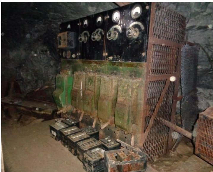
An array of battery chargers found at the foot of Olwyn Goch Shaft, power for the mine's locomotives
